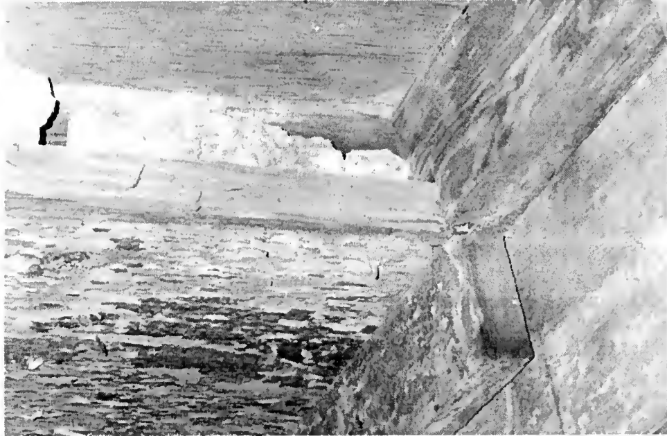
Figure 25 Close-up of “Palling” under the floorboards in the Basement of the South Wing of the Main House, 2002
